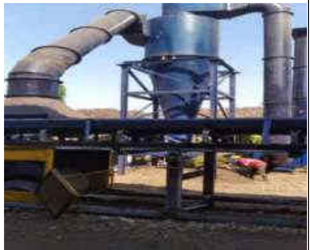
Cyclone separator (removal of fine plastic from soil)
