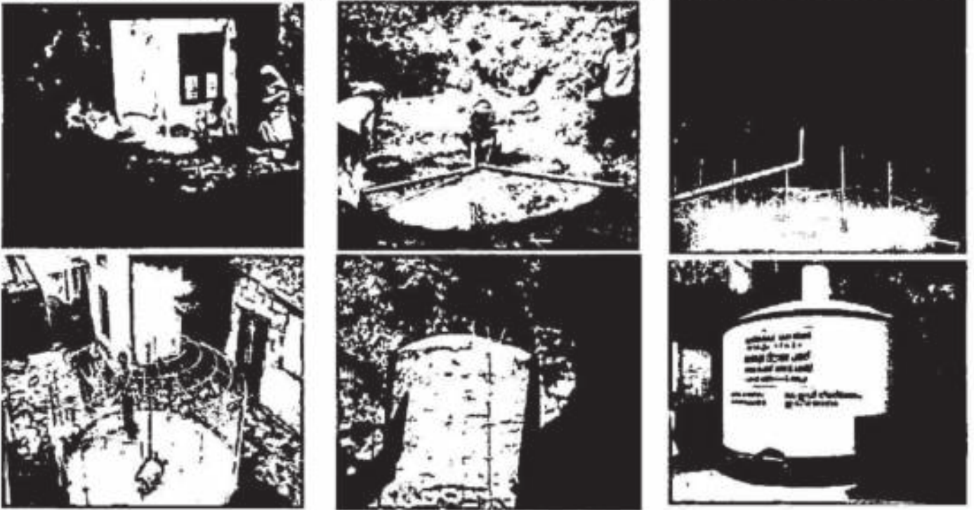
Various stages of construction of Rain Water Harvesting Tank of 10000 Litres capacity.
